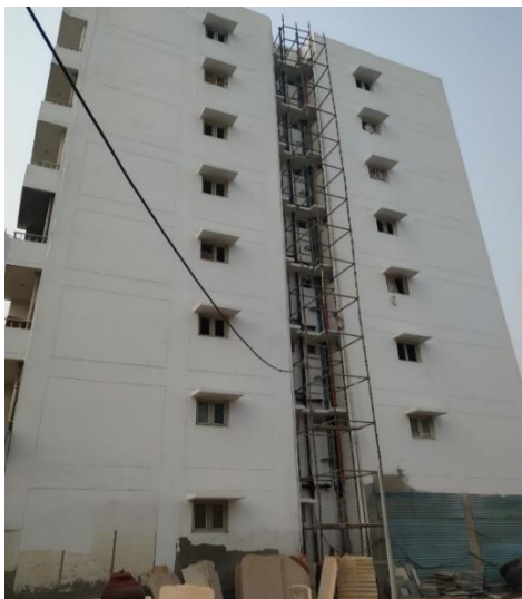
Picture Shows 768 Bedded Hospital at Burari which was Supposed to be Functional by June 2019 but is yet to
