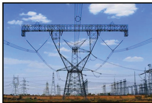
World's Highest Voltage 1200 kV UHVAC Station at Bina, Madhya Pradesh.
